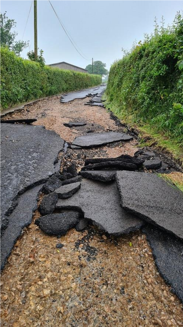
Figure 35: Road damage in Whitestaunton. Photo from Access restored as Highways teams respond to flash flooding damage | Somerset County Council Newsroom ( somersetnewsroom.com ).
